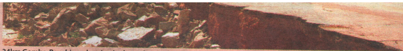
34km Gombe-Bauchi road caving in due to heavy downpour
