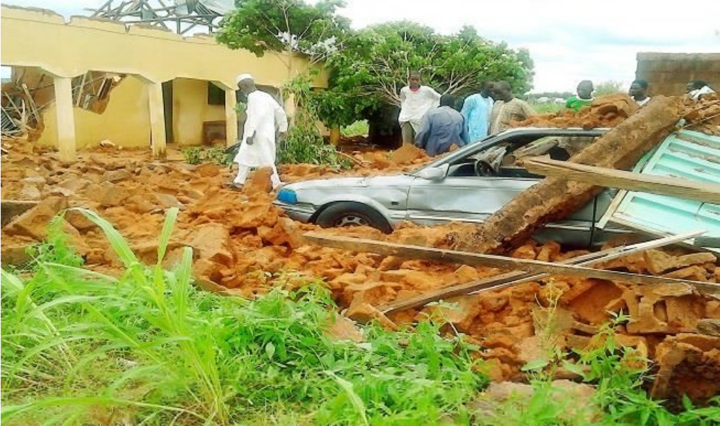
Damage caused by a windstorm at Shuni town of Dange-Shuni Local Government Area of Sokoto State yesterday Photo: Abubakar Auwal
