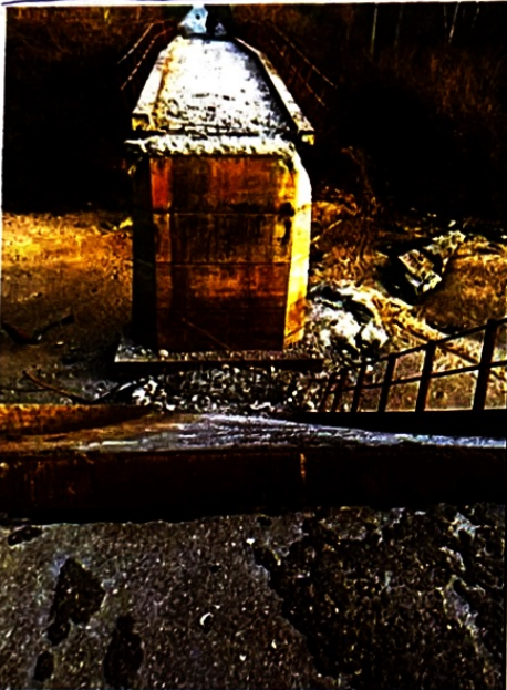
•The bombed Lunma-Babana bridge, in Borgu local government area of Niger State.
