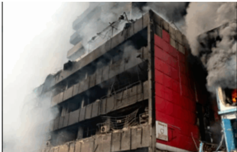
Fire-ravaged Great Nigeria Insurance House on Martins Street, Lagos Island. Credit: Lagos State Fire and Rescue Service | X
