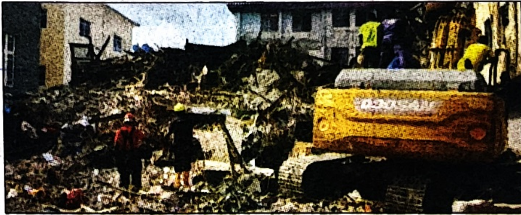
•Site of the collapsed building. Photo: Johnson Idowu
