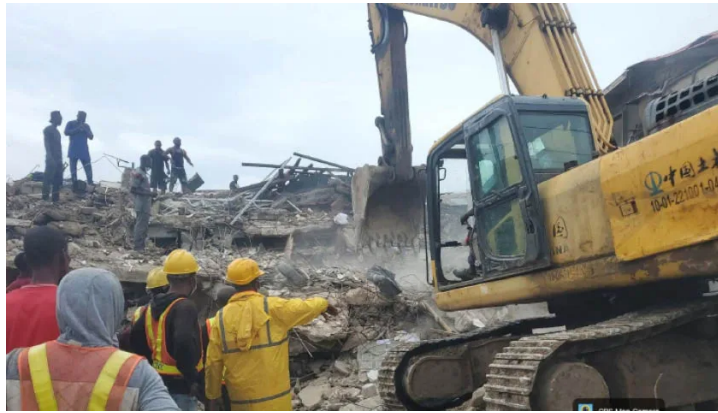
Rescue operations at the scene of a building that collapsed at Alakija area of Lagos State yesterday Photo: NEMA
